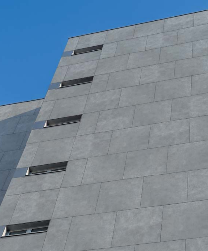
Facade: MATERIA Re_Tour Fog FullBody3D bocc.
